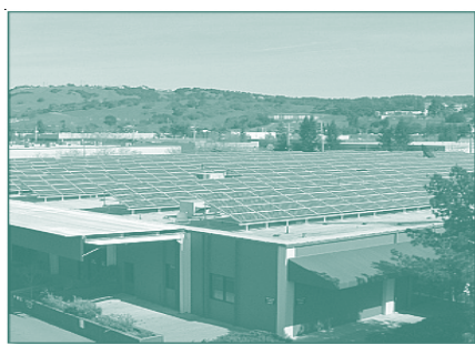
200 kW of solar on top the Pine Creek Properties. Image: Sharp Solar
